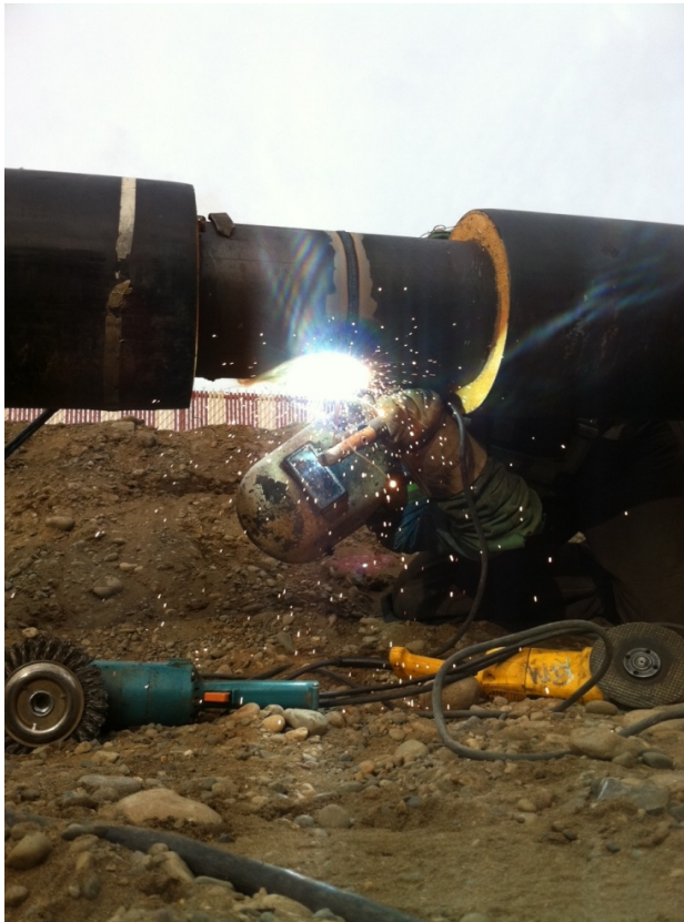
Some of the piping for the Downtown District Energy System being welded together. (Photo courtesy Kristy Brown)
